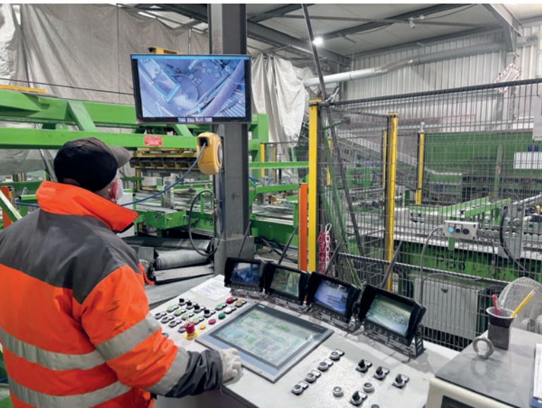
Everything in view: Control panel of the sorting and packaging system
